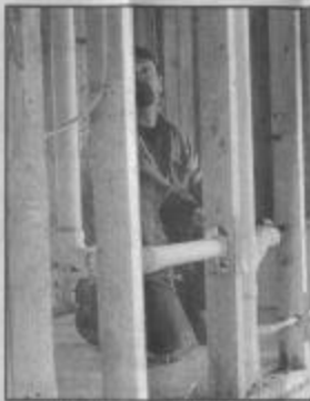
Elizabeth Robertson/Philadelphia Inquirer Buyers can use the pre-drywall inspection to see where wiring, pipes and ducts are — handy knowledge for future remodeling.
